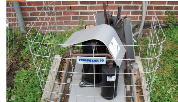
Air-conditioner damaged by copper thieves.
